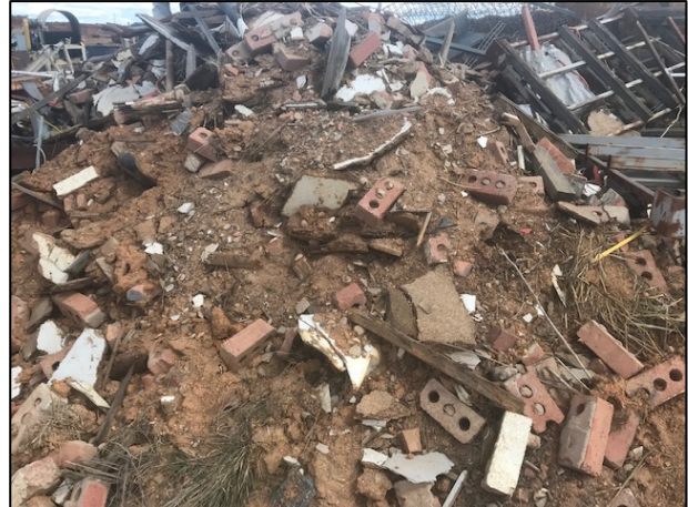
Stockpile containing bricks, chipboard and scrap metal requiring removal
